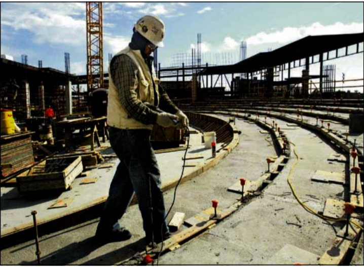
Rodolfo Gomez works on the upper orchestra level of seating in the performing arts center's concert hall. The center is to open in fall 2005.
